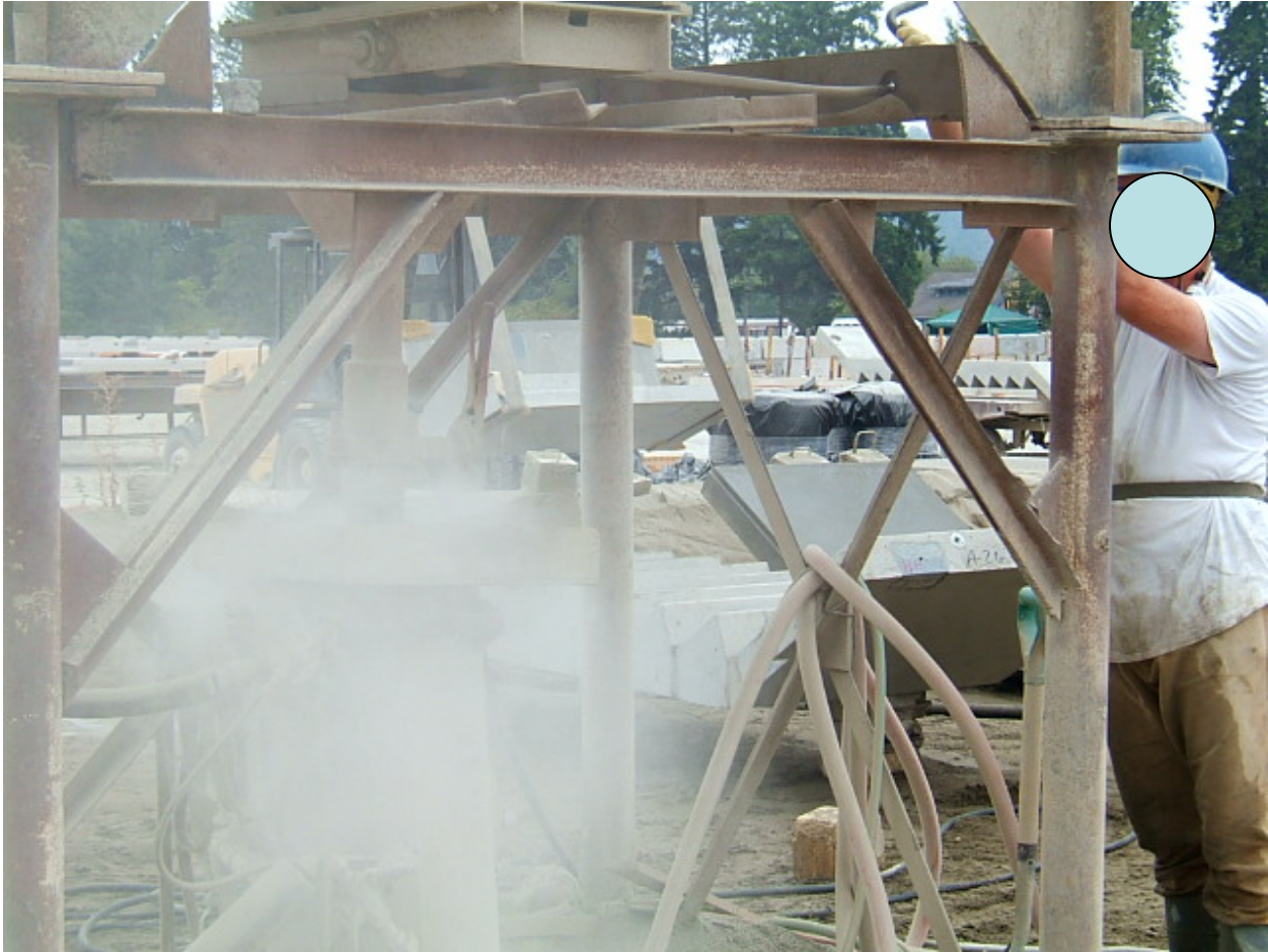
Figure 10. Filling the abrasive blasting pot with dry sand creates obvious dust emissions. The sand flows by gravity through a chute into the abrasive blasting pot. The workers are generally able to avoid the dust plume. The purchase specification on the sand limits the fines content (sand passing through a 100-mesh screen) to less than 3% by weight.
