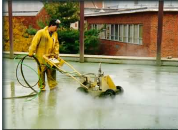
Figure 4. Ultra high-pressure water is used to clean concrete surface on a parking ramp. (Photograph courtesy Jet Edge). Apparently the use of water greatly suppresses the dust generation.
