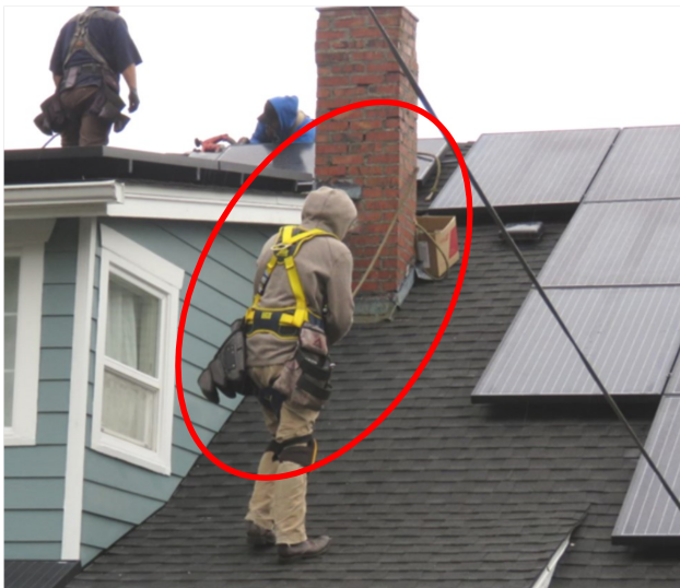
Fig. 4 This chimney obstructs the movement of the workers and reduces resistance capacity of the safety line
