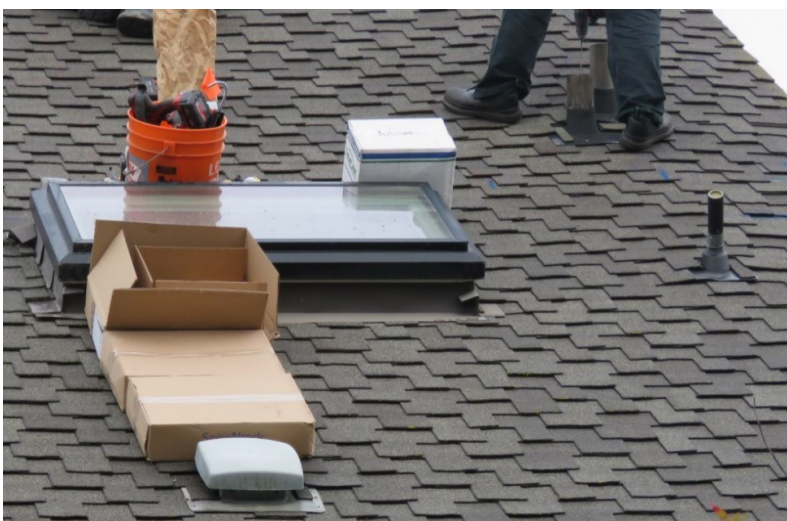
Fig. 5 This skylight and exhaust vent prevent installation materials from sliding, while the small drain vents pose high tripping hazards for the worker
