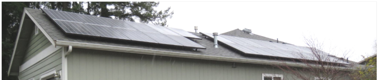
Fig. 6 This solar energy system is divided into two arrays to avoid the existing chimney
