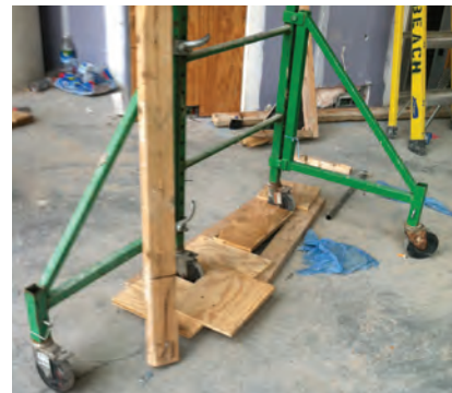
Figure 3: Improperly secured base on mobile scaffolding
