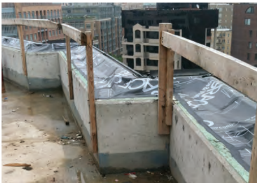
Figure 1: Unprotected roof edge
