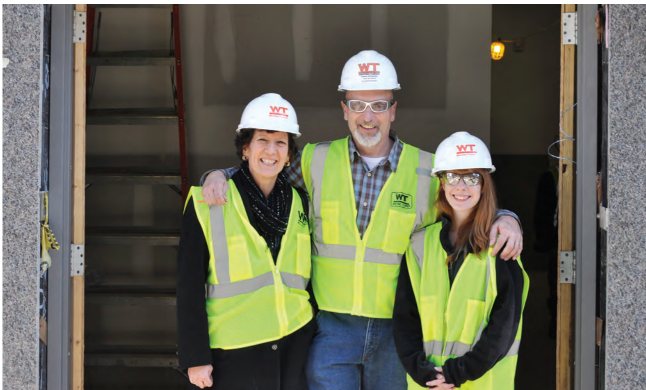
Project Principal Investigator Dr. Melissa Perry, Site Superintendent Mike Whitmore, and Student Researcher Amanda McQueen at the construction site.
