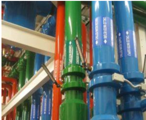
Pipe identified by color (blue: potable cold water, green: hot water, and red: fire water) www.safetysign.com/blog/brimar-is-coming-to-the-ahr-expo/ visited by Briones on 11/02/2017
