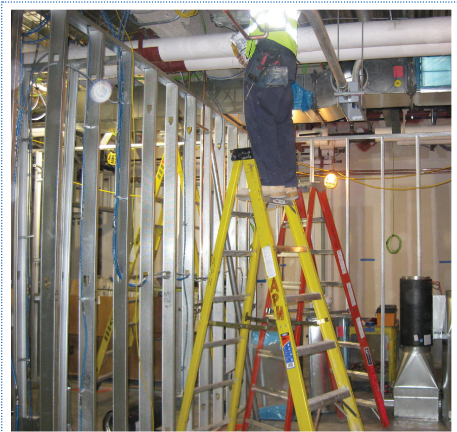
Unsafe posture. Worker should be on a lower rung; a taller ladder is needed.
