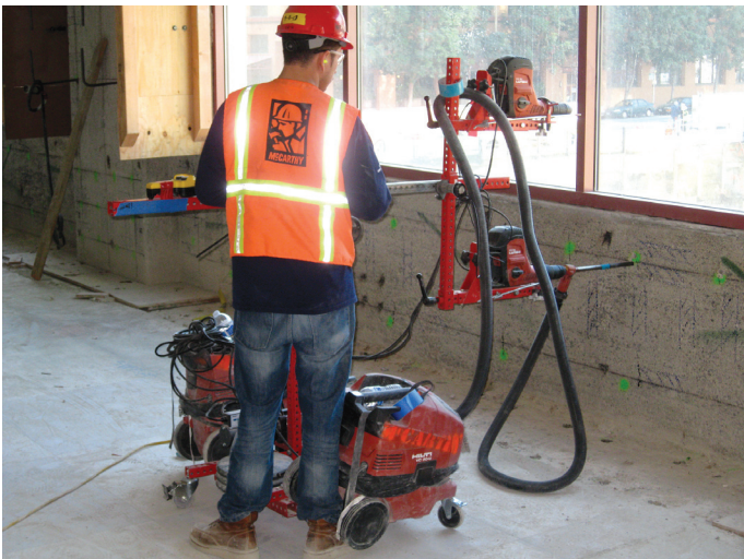
Laborer at a San Francisco site using drilling jig set up for 2 drills but only drilling with one. Concrete dust is captured during drilling with a new hollow bit system.
