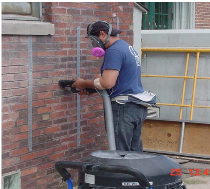
Figure 1. A vacuum cleaner exhausts air from a hood mounted on a grinder used for mortar removal.
