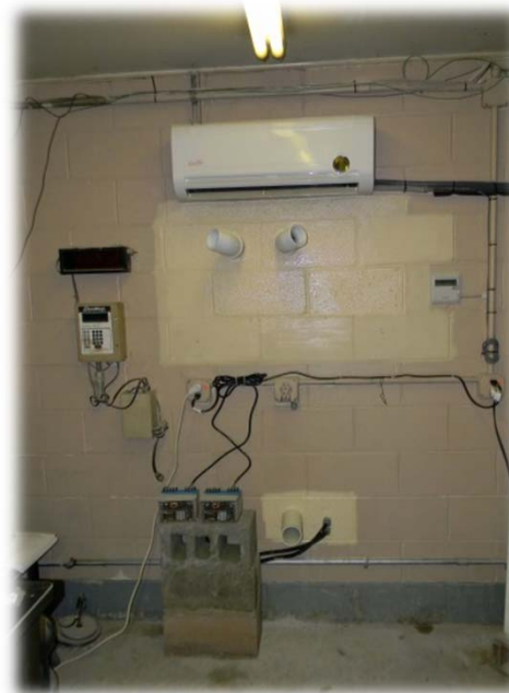
Control Room - surface facility (New Jersey)
