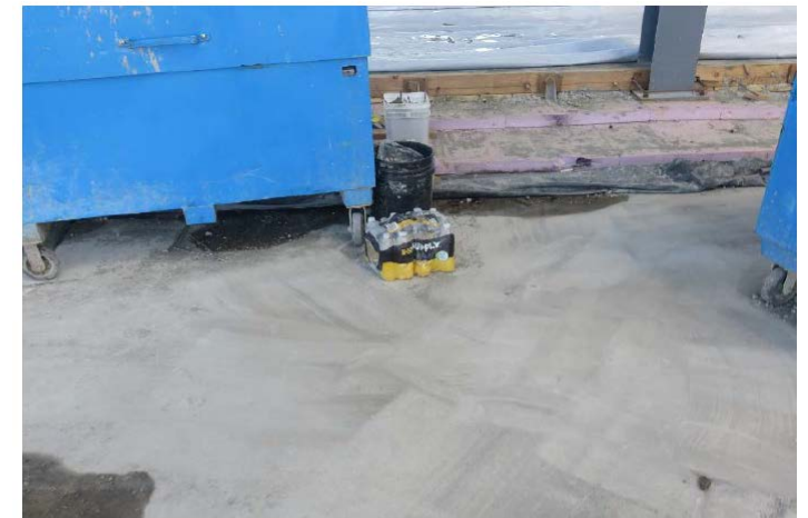
Photo 3. Area where the apprentice ironworker went to retrieve a bottle of water when he was struck by the dropped steel wedge.
