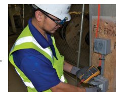
Worker testing a circuit to ensure that it is de-energized
