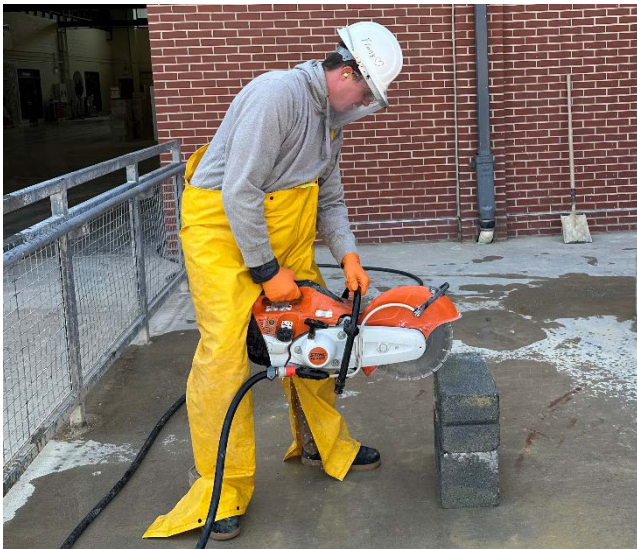
Worker uses a cut-off saw to cut concrete blocks Photo Credit: International Union of Bricklayers and Allied Craftworkers
