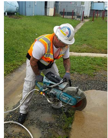
Worker uses a handheld power saw with integrated water delivery system. (Photo Credit: OSHA)
