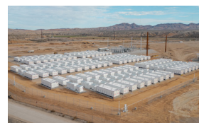
The Reid Gardner Battery Energy Storage System in Nevada.
