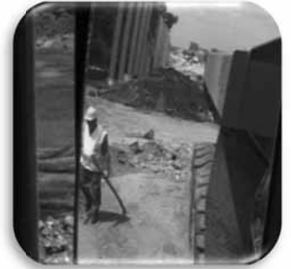
Adjust and clean mirrors; check back-up alarm.
