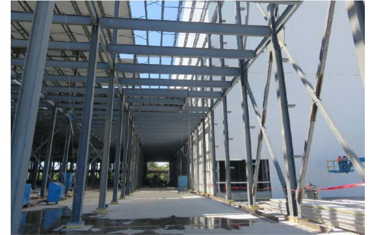
Photo 2. Interior view of incident scene at the cold storage facility under construction.
