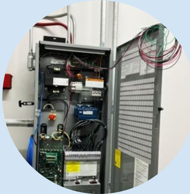
Open Panels, Switchgear, Testing & Commissioning
