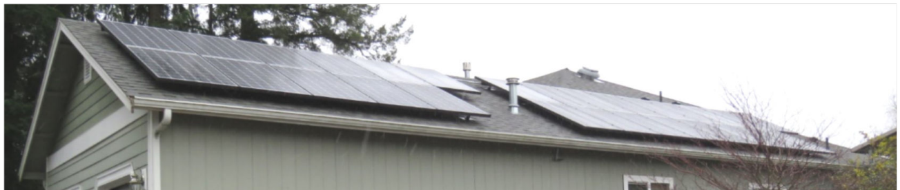
Fig. 6 This solar energy system is divided into two arrays to avoid the existing chimney
