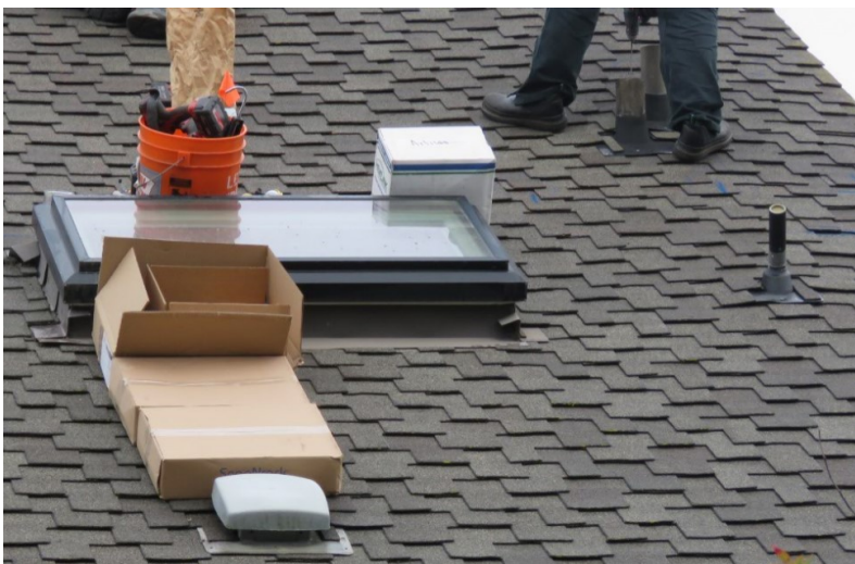
Fig. 5 This skylight and exhaust vent prevent installation materials from sliding, while the small drain vents pose high tripping hazards for the worker
