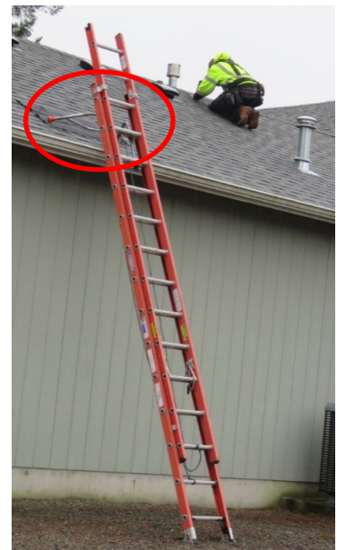
Fig. 14 Ladder with a ladder safety device
