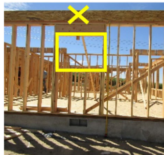
Framer fell from rim joist (x) above window opening to floor deck.
