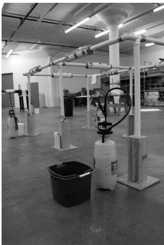
You will learn how to remove ACM from a pipe using a glovebag...
