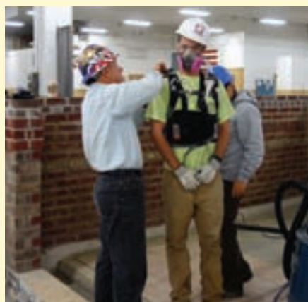
NIOSH researchers set up the new Helmet Cam technology on BAC Local 18 OH apprentice Caleb DeLaVega before he begins tuckpointing.
