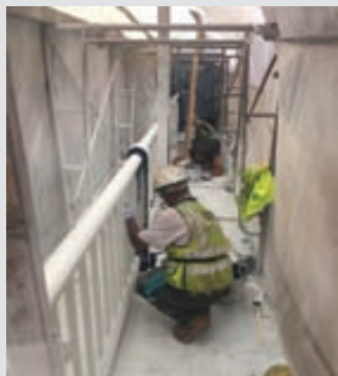
Painters applying an isocyanate-based top coat inside an enclosure on a highway bridge.
