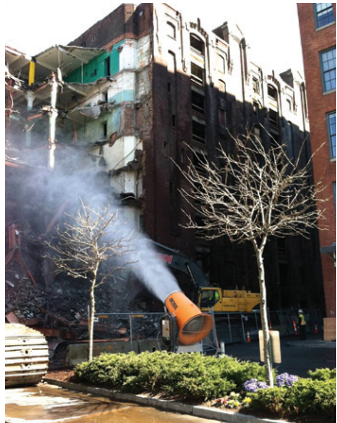
The manufacturer of the Dust Boss water cannon and a demolition contractor joined with researchers to evaluate dust and silica reduction from this water suppression method.
