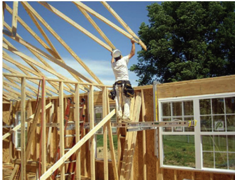
Carpenter guides roof trusses into place while using a Wall Walker, a hanging scaffold system with a walking surface hung from braced walls of a home. If used over 6', guard rails must be installed.
