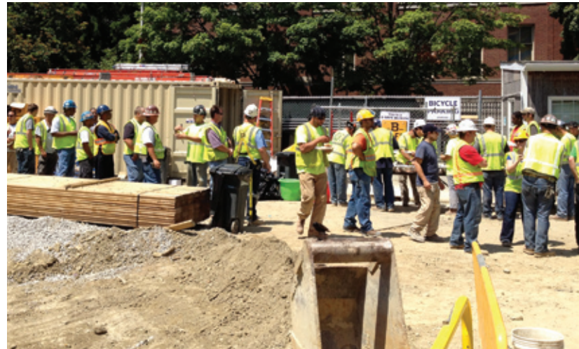
The Building Safety for Everyone program measures and scores a site's safety performance among its many subcontractors. When the scores make the grade, as they did at this intervention site, workers receive a safety recognition lunch. A program focus is positive reinforcement for safe work practices.
