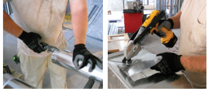
In a test of tools (manual hand crimper vs. a powered crimper attachment designed for a cordless drill) to crimp the edge of a small round duct pipe, researchers found that the power tool performed the job faster and better, and with less hand effort for the worker, than the manual tool.
