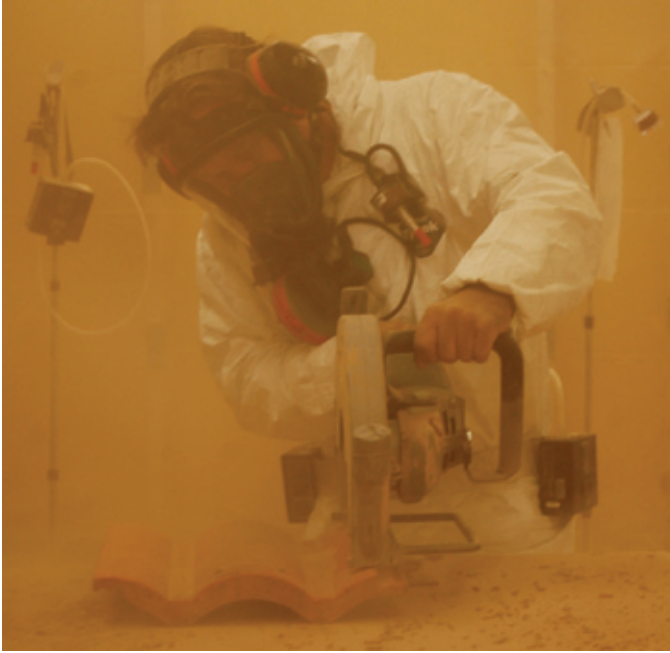
Although researchers were collecting data on worker exposure to nanotubes in roof tiles, the demonstration photos show the obvious: cutting roof tiles creates a thick haze of dust, which includes silica along with other fine particles, unless engineering controls are used.
