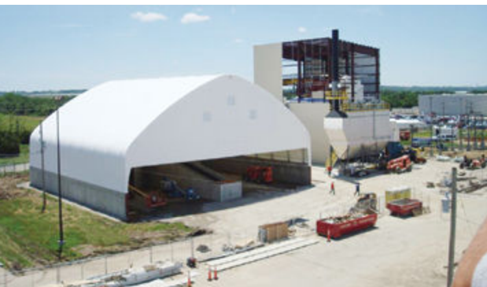
Fabric structures have the room, strength, capacity and safety that's required for any major jobsite. (Photo provided by Clearspan Fabric Structures)
